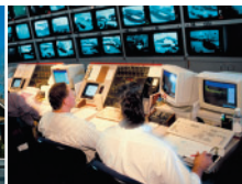
Security and Surveillance
