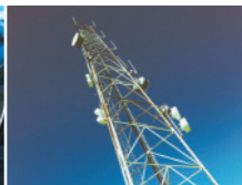
Voice and Data Backhaul
